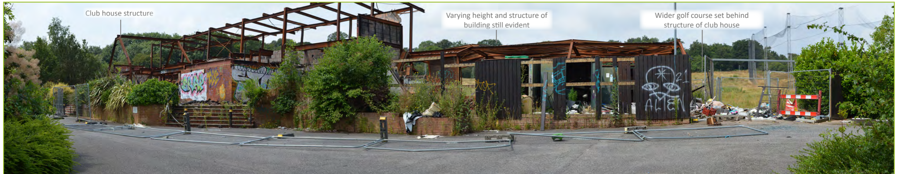
Image E: Derelict clubhouse building
