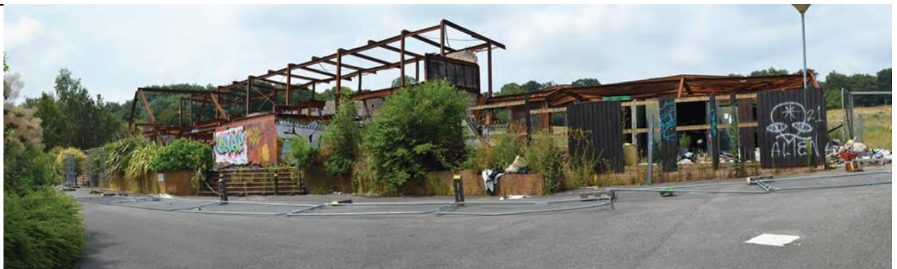
Figure 2: Fire Damage and Graffiti to Clubhouse Building
